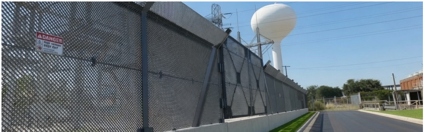
ENC composite fence on an energized site. No conductive path from the fence to grade.
