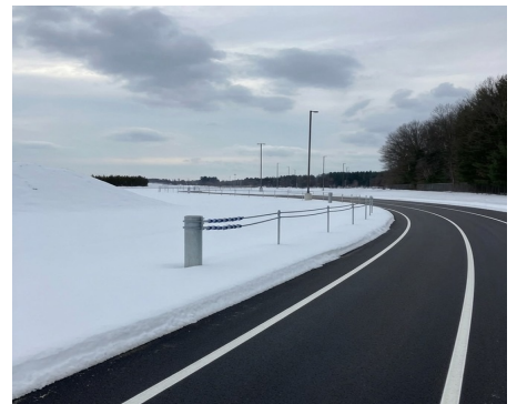
Barnes Air National Guard Base — roadside curve, freeze-thaw.
