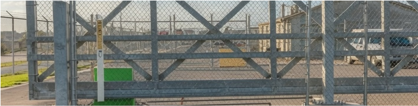
Electrically operated crash gate on a secured facility entrance, carried on a ground track across the opening.
