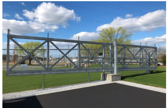
Galvanized crash gate at a utility substation. The trussed frame carries chain link infill.
